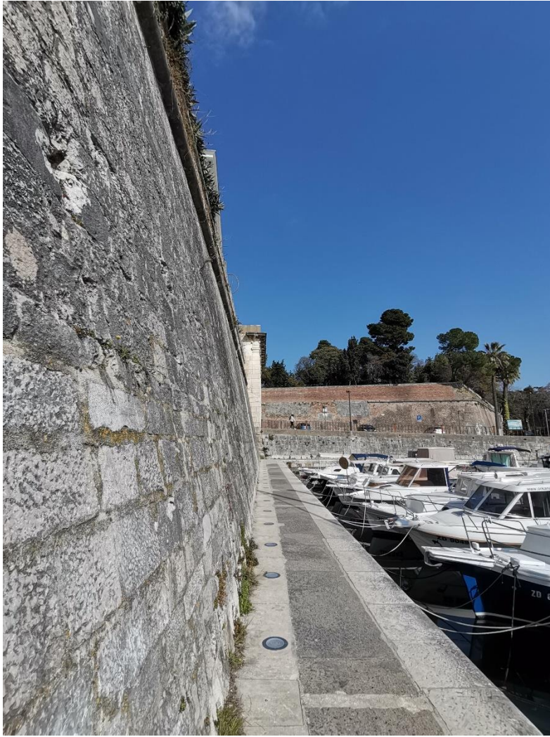
Figure 19. Zadar, view of the elongated Bastion Ponton and the corner of Porta Terraferma. Photographed by Karla Papeš.
